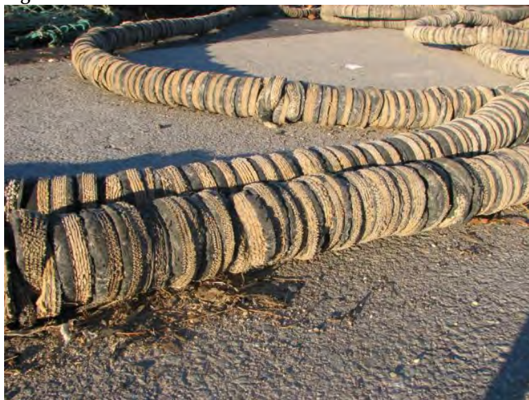
Figure 3 - Ground cable with cookies
